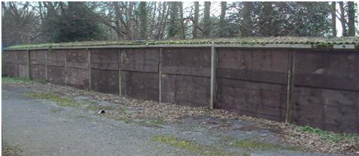
Before: Boarded up garages
